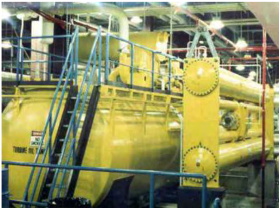
Figure F-3. The lube oil tank below the turbine deck.
